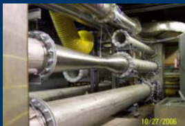
West Virginia University's SSV-CVS Installed at the CAFE Engine and Emissions Testing Laboratory
