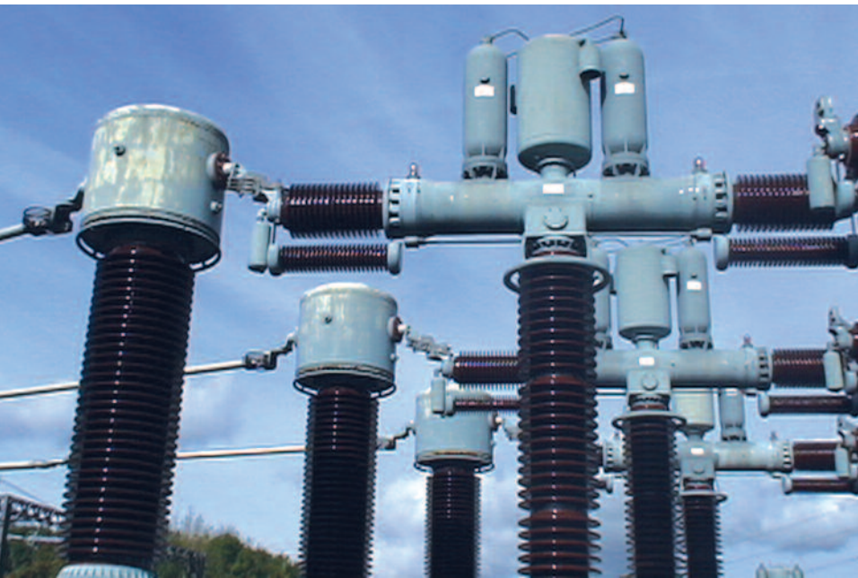
High voltage switchgear
