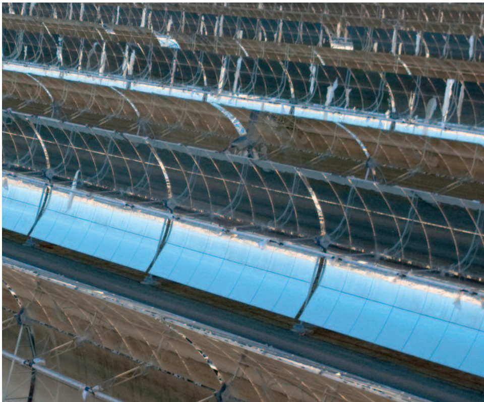
A parabolic trough power plant
